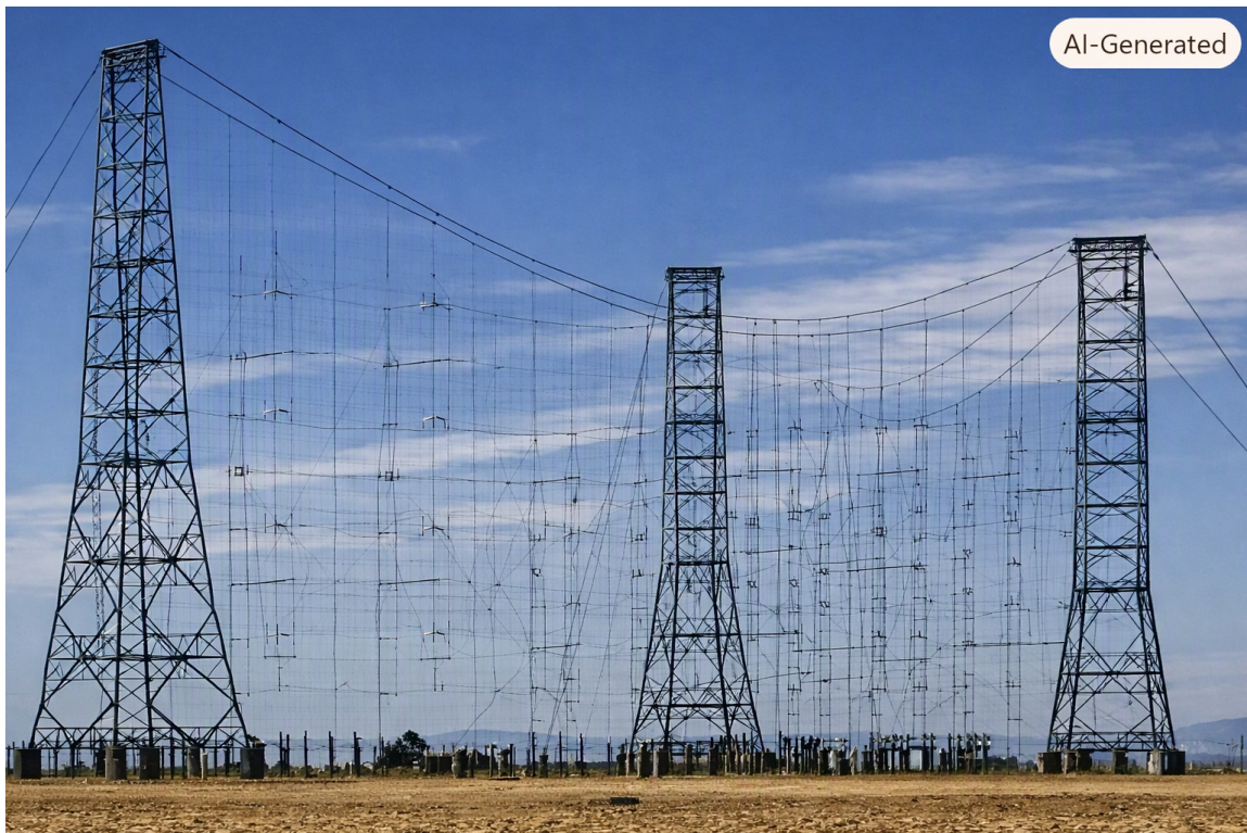
Above Photo Enhanced — Four Bays of Two Dipole Columns per Curtain Left Tower to Center Tower: 700 ft. — Left Tower 325 ft. — Center Tower 305 ft. Taken from Radio Station Road, Dixon, CA (Photo Courtesy of Stephanie Arrich)
