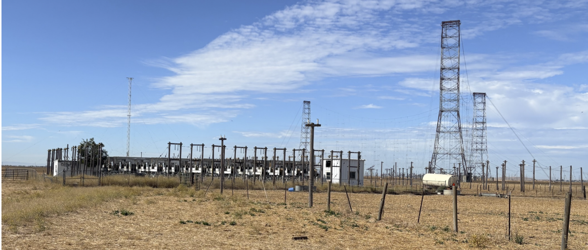
Switch Matrix and Dummy Load Shed (Photo Courtesy of David Arrich, AD6AE)
