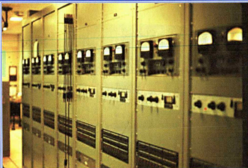
Control room racks, One rack for each transmitter Gates Modulation monitor, UREI audio limiter, Kahn Symetrapeak .
