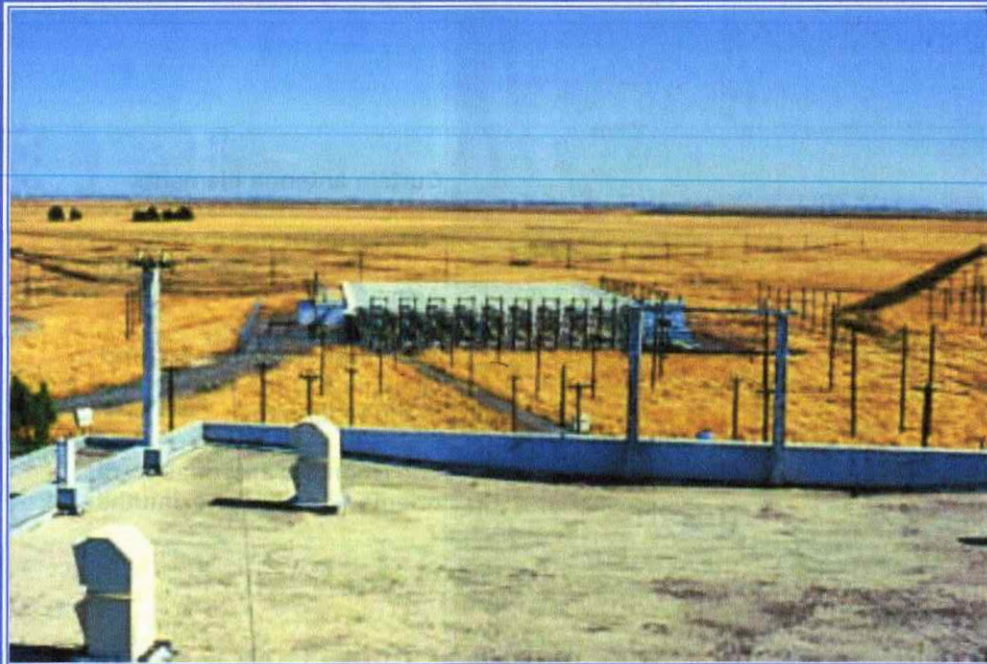
Antenna switchbay matrix
